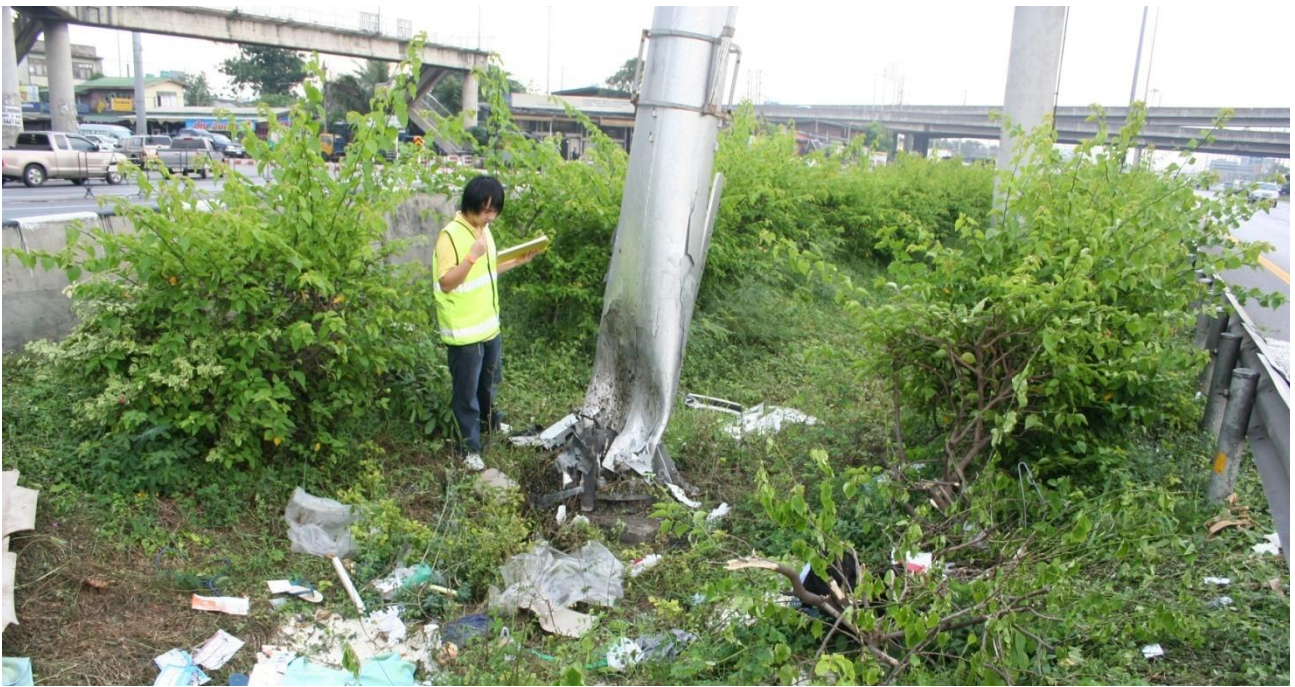
Figure 3-6: High Mast Lighting after Crash
