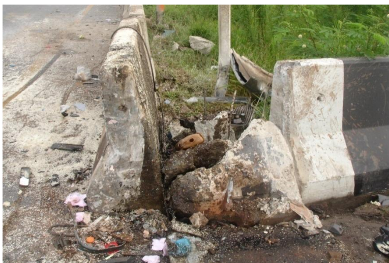
Figure 3-9: Damaged Concrete Barrier
